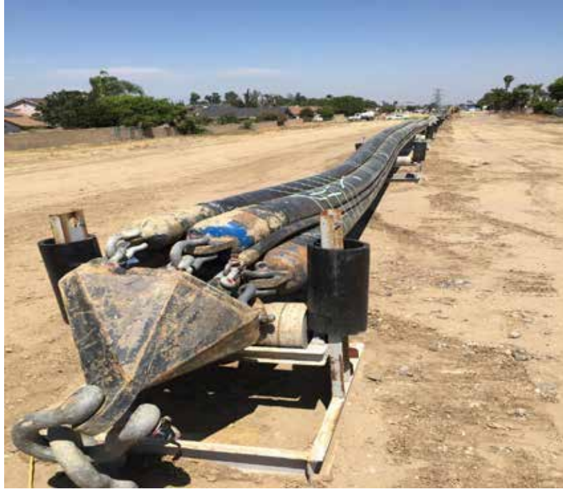
Large underground and undersea HV and EHV cable projects like this project at SCE are becoming more common in the T&D industry.
