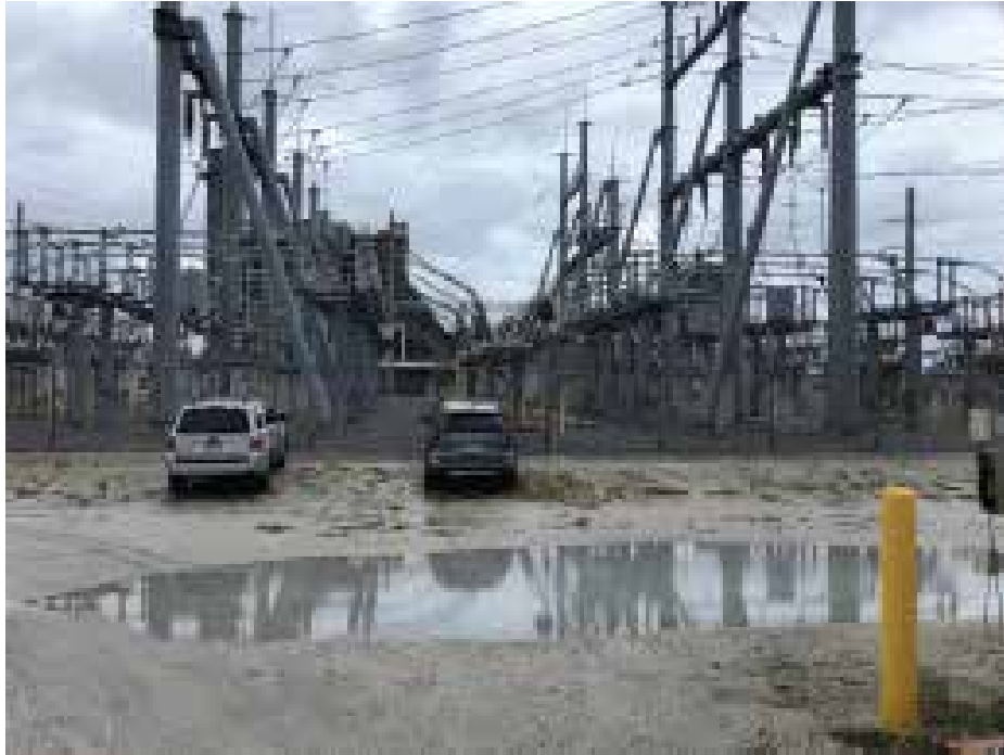
An upgraded and hardened substation will be a key part of a new, reimagined microgrid.
